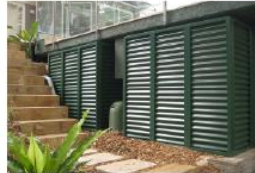
Figure 322. Concealed tanks integrated with the design.
